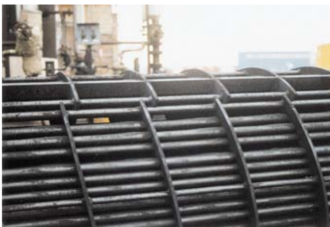
FIG. 12 Replacement helically baffled heat exchanger bundle, inspected at annual turnaround after one year of operation in bitumen service.
