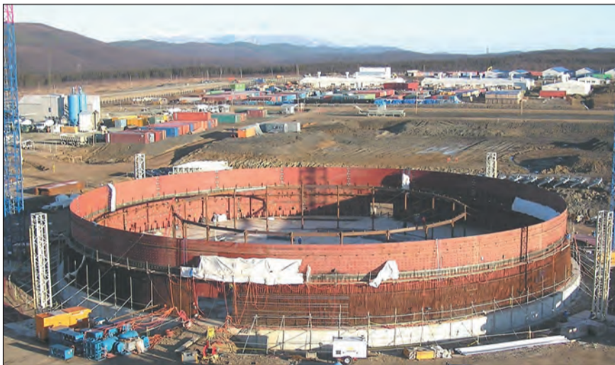
Figure 1: The initiation of steel construction on the first LNG tank in Sakhalin
