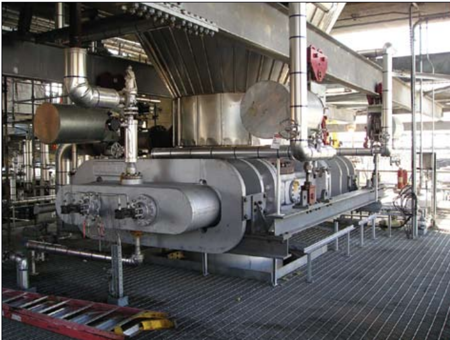
Shown are the open design and monorail system of the bottom unheading valve (Fig. 4).
