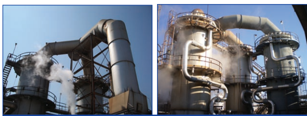
Figure 1. Existing two cylindrical reformer hydrogen unit (left) revamped by the addition of a third cylindrical reformer (right).
